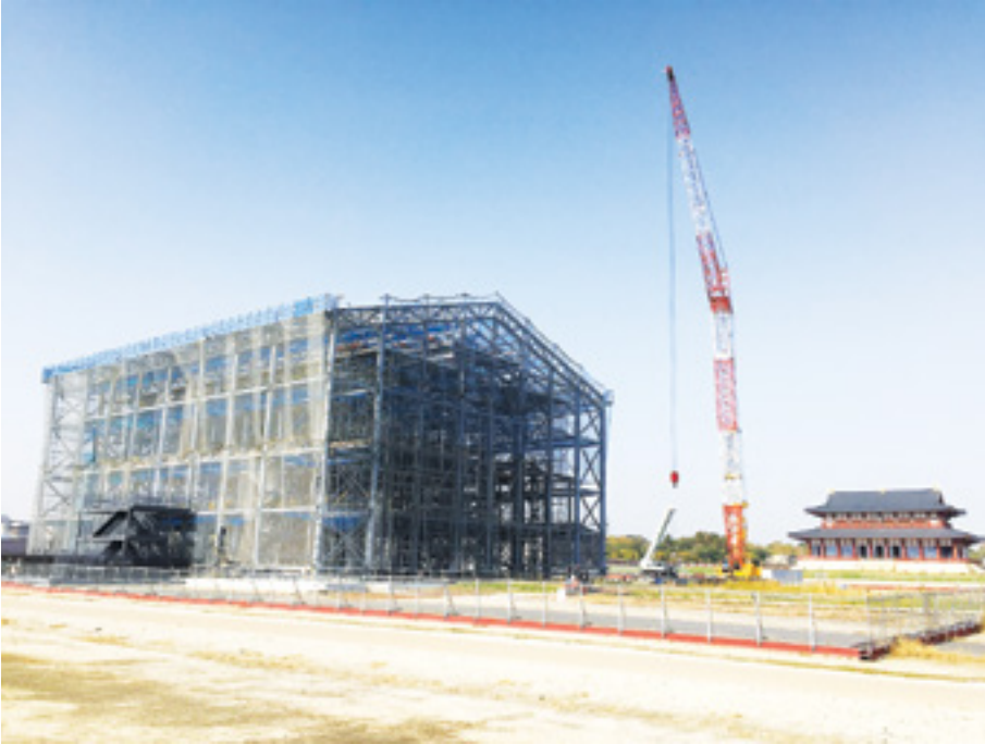
Figure 5. Heijō Palace. Reconstruction work on the Daigokumon. Source: Photo by Jens Sejrup, 2018.
